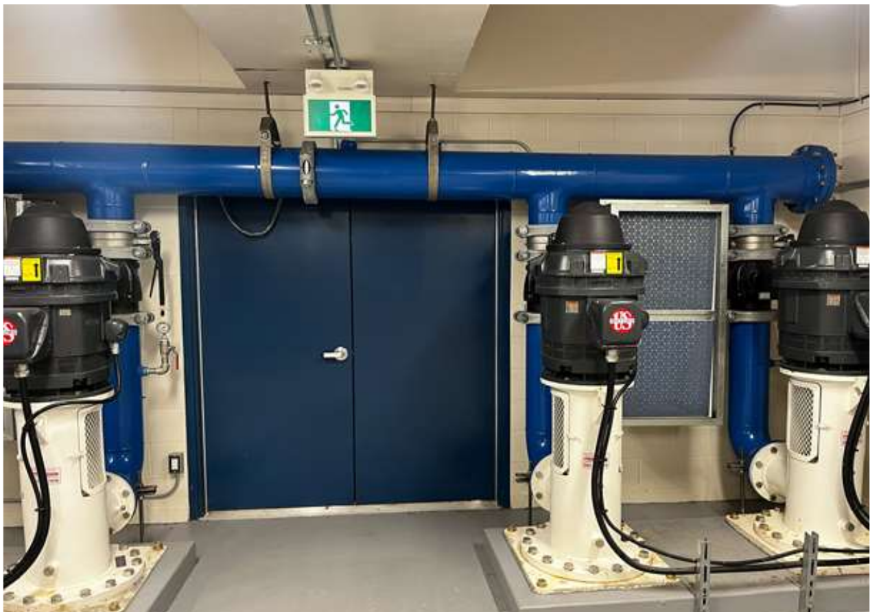
Schikurski Park Booster Station
