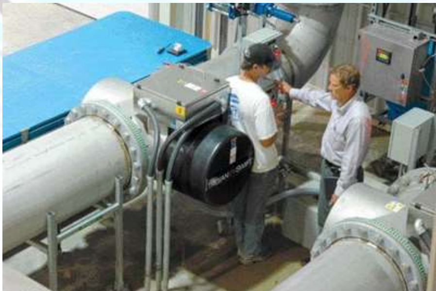
Arrow Creek Ultra Violet Disinfection Equipment
