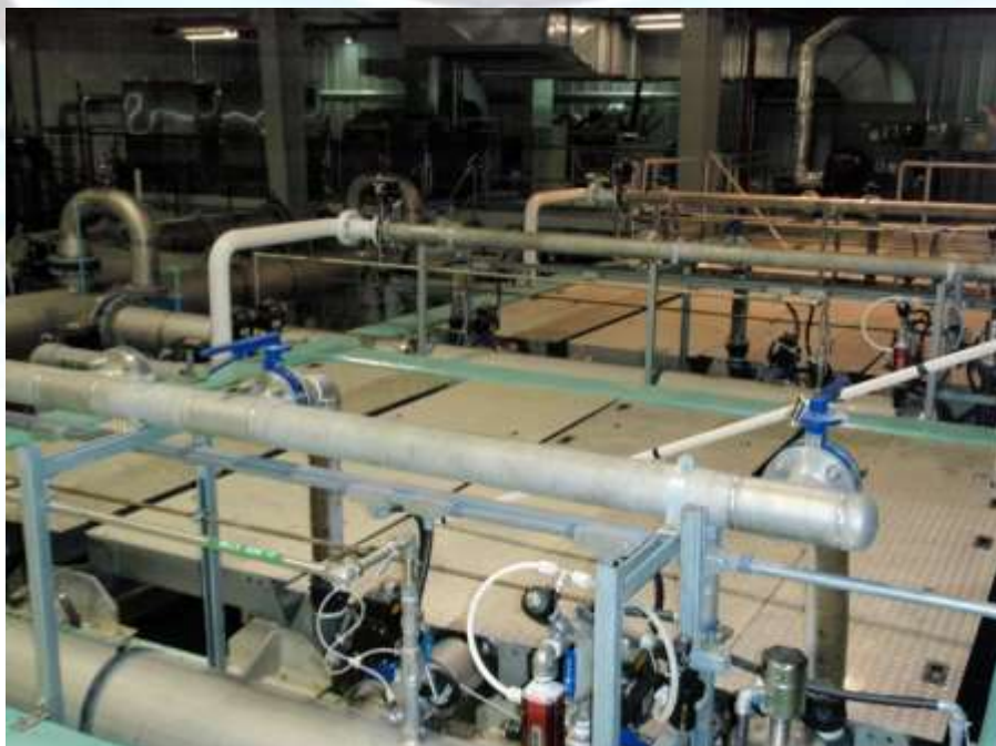
Arrow Creek Water Treatment Plant
